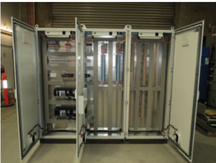
One of the NCS Master PLC Panels ready for Factory Testing, in excess of 20 of these produced for the project
